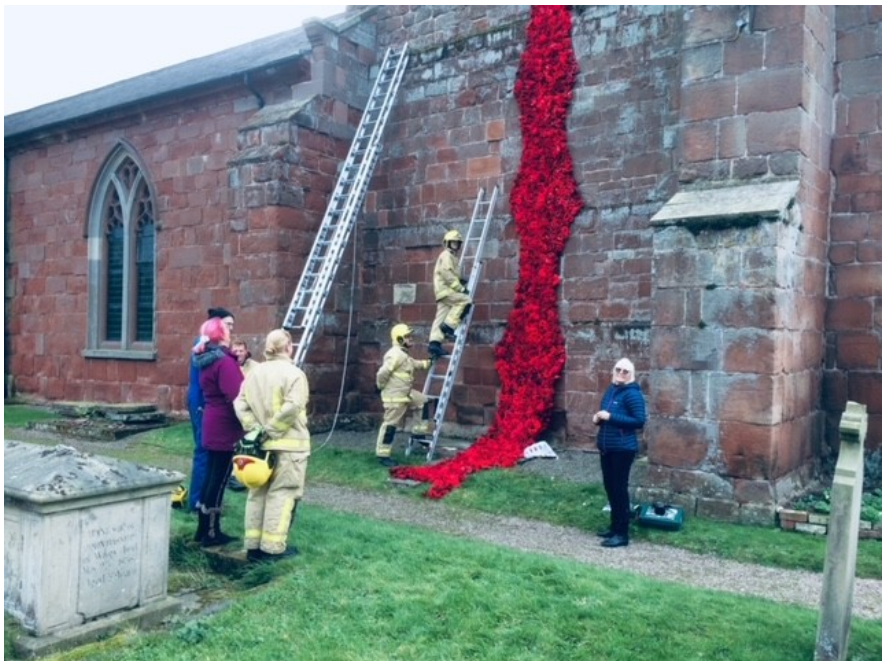
Thanks to John Russell for these photographs of the poppies being installed on All Saints' tower by the Fire Service.
